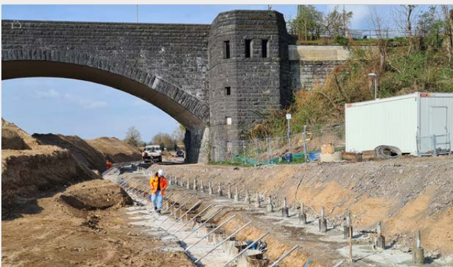
Good drilling progress was maintained despite the limited clearance beneath the bridge.
