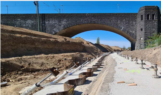
TITAN micropiles were installed to anchor the sheet pile wall and as foundations for the retaining wall.
